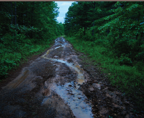
Weak road base material and construction lead to erosion and poor driving conditions
